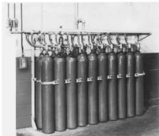
FIGURE A.4.6.5.2 A Typical High-Pressure Storage Facility.
